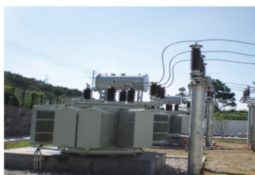
Reactor shunt BKS-60000/35 funcionando en la provincia de Anhui BKS-60000/35 Shunt Reactor in Anhui Province
