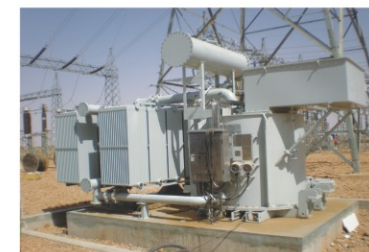
Reactor Shunt BKS-15000/11 de Funcionando en Sudan NEC BKS-15000/11 Shunt Reactor in Sudan NEC
