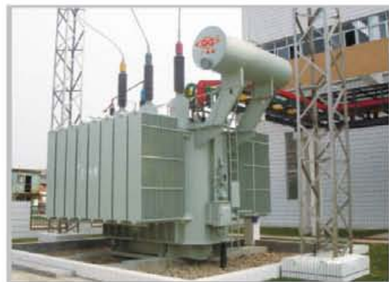
广州员村变电站110kV主变 Operating in Guangzhou substation 110kV main transformer
