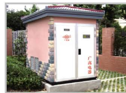
广州华南碧桂园欧式变电站 Operating in Biguiyuan prefabricated substation
