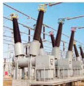
Sf6 Circuit Breaker
