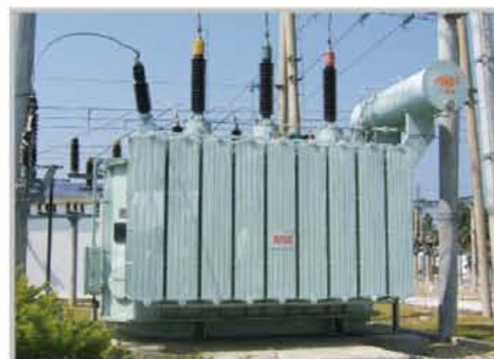
湖南沙田电站110kV主变 Operating in Hunan substation 110kV main transformer
