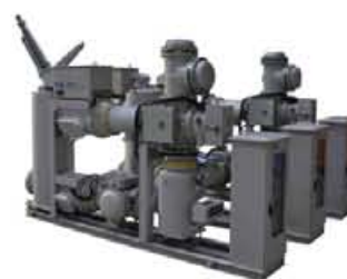
GIS (Gas Insulated Substation)
