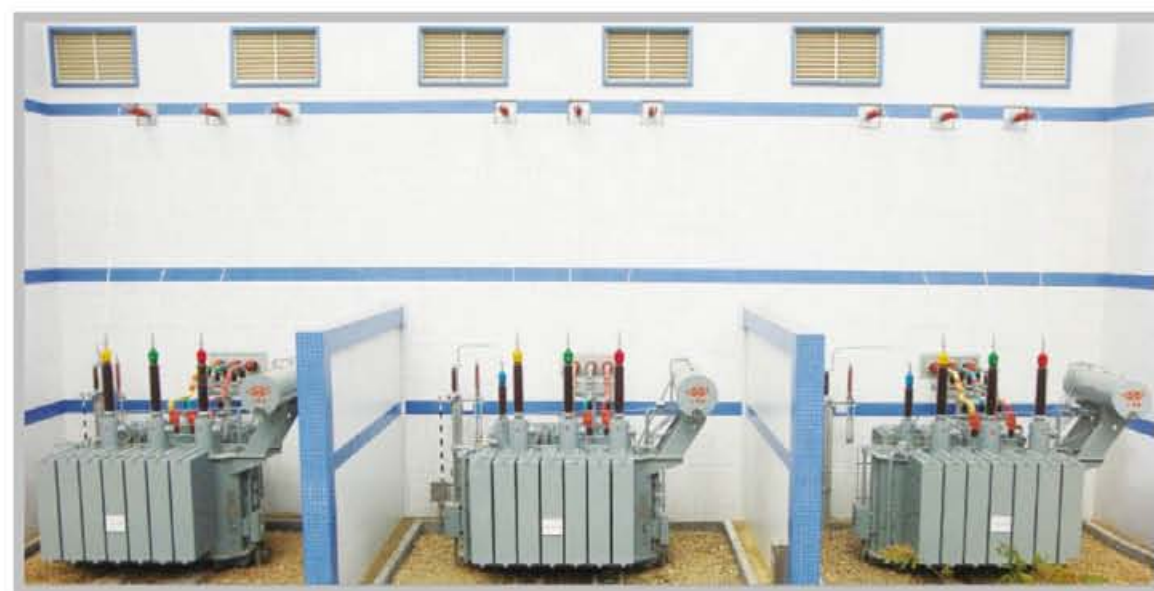
东莞供电局新厅变电站110kV主变 Dongguan power supply bureau Xinting substation 110kV main transformer
