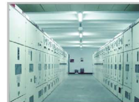
高压开关柜XGN XGN high-voltage switch cabinet
