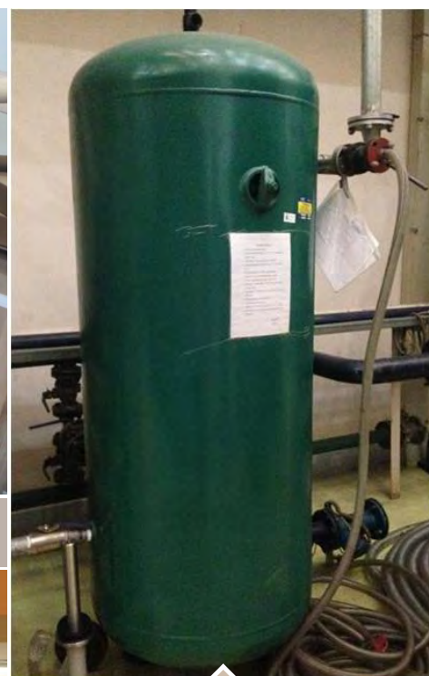
The site is equipped with dry air generator. Dry air with dew point \leq -70^{\circ}\text{C} is generated to reduce the degree of moisture absorption when the active part is exposed to the air.
